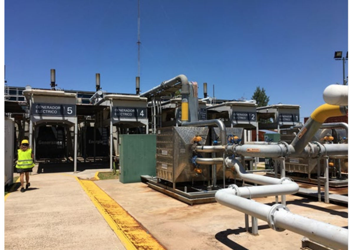
Large Power Generation Plant Operating on Landfill Gas (MSW Landfill in Buenos Aires)
